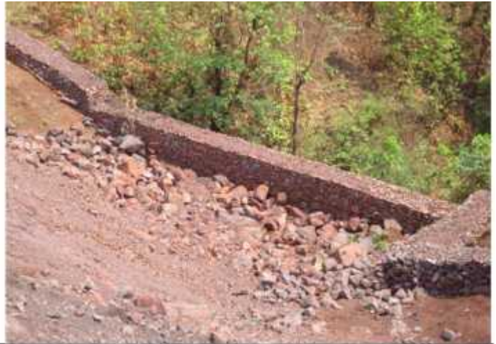
PHOTO # 2: SHOWING RETAINING WALL ALONG WITH GARLAND DRAIN ALL ALONG THE DUMPS
