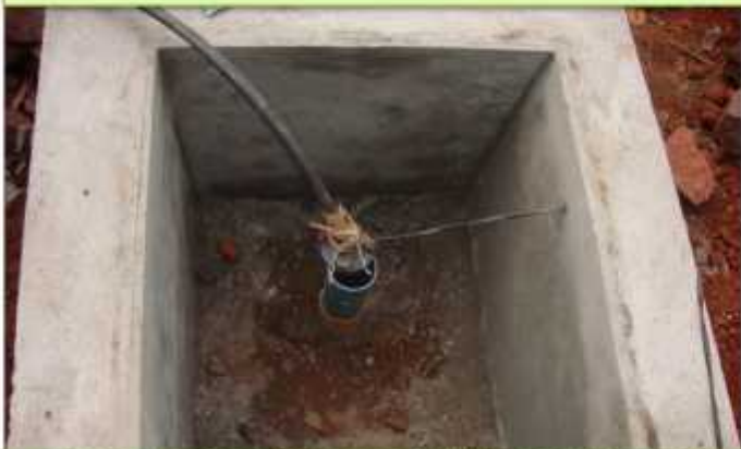
PHOTO # 11 SHOWING BORE WELLS PROVIDED FOR VILLAGERS
