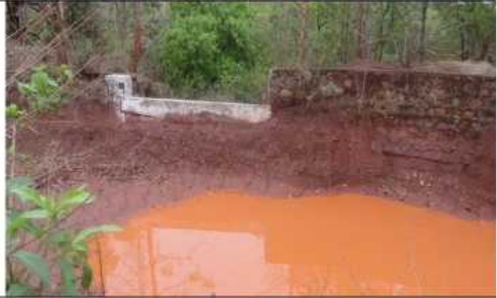
PHOTO # 4A: SHOWING CHECK DAM CUM SETTLING PIT BEFORE FINAL DISPOSAL TO OUTSIDE WATER BODIES
