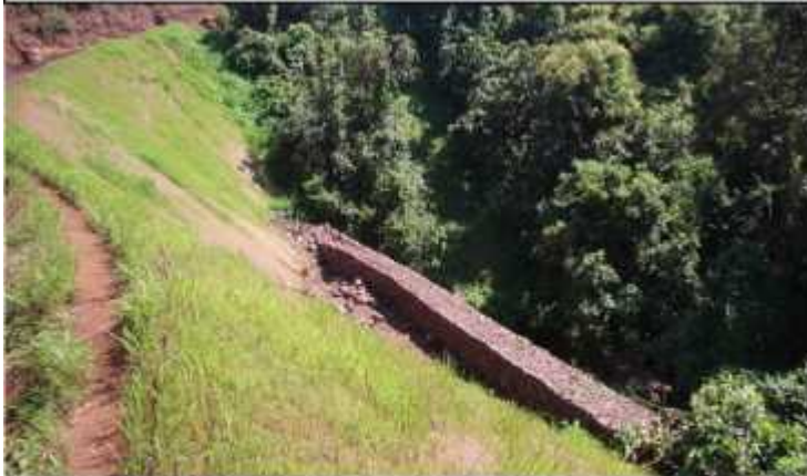
PHOTO # 3 SHOWING THE DUMP STABILIZATION WITH COIR MATTING, RETAINING WALL FOLLOWED BY GARLAND DRAIN
