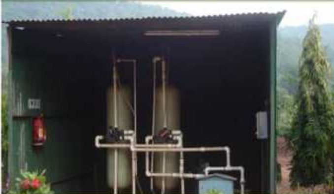
PHOTO # 7 : SHOWING THE STP FOR TREATMENT OF DOMESTIC EFFLUENTS
